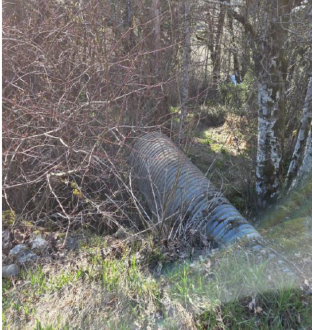
Exhibit 5. this pipe face to my farm, and creek water from this pipe flooding my land every year. Although it is located at property 450.
