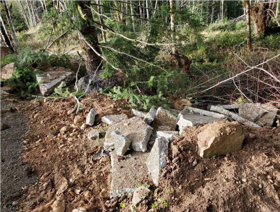
Construction debris at uppermost landing. Debris pushed in drainage channel.
