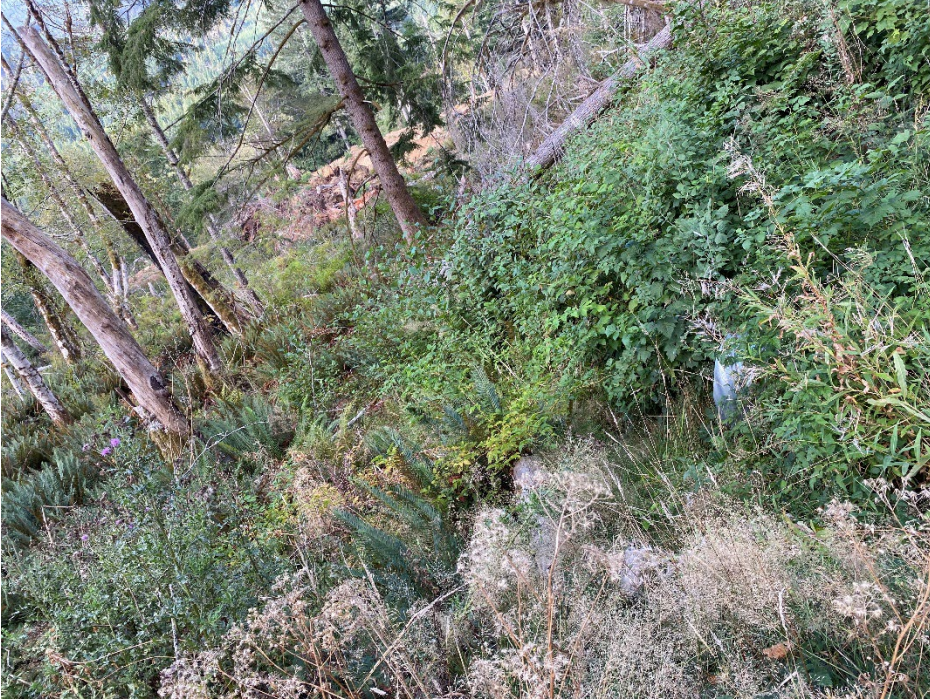
Looking south toward Franklin River Road at culverted drainage downstream at uppermost landing.
