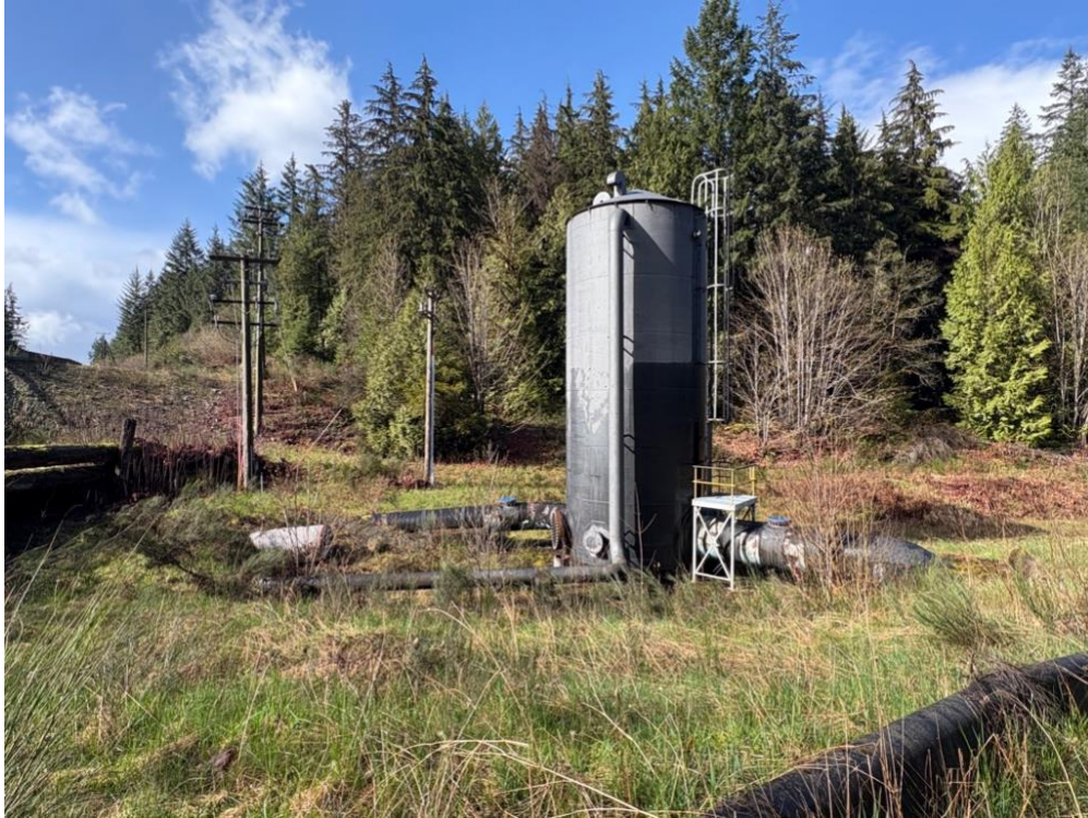
Figure 2. Catalyst / Domtar water storage located near Sproat Lake.
