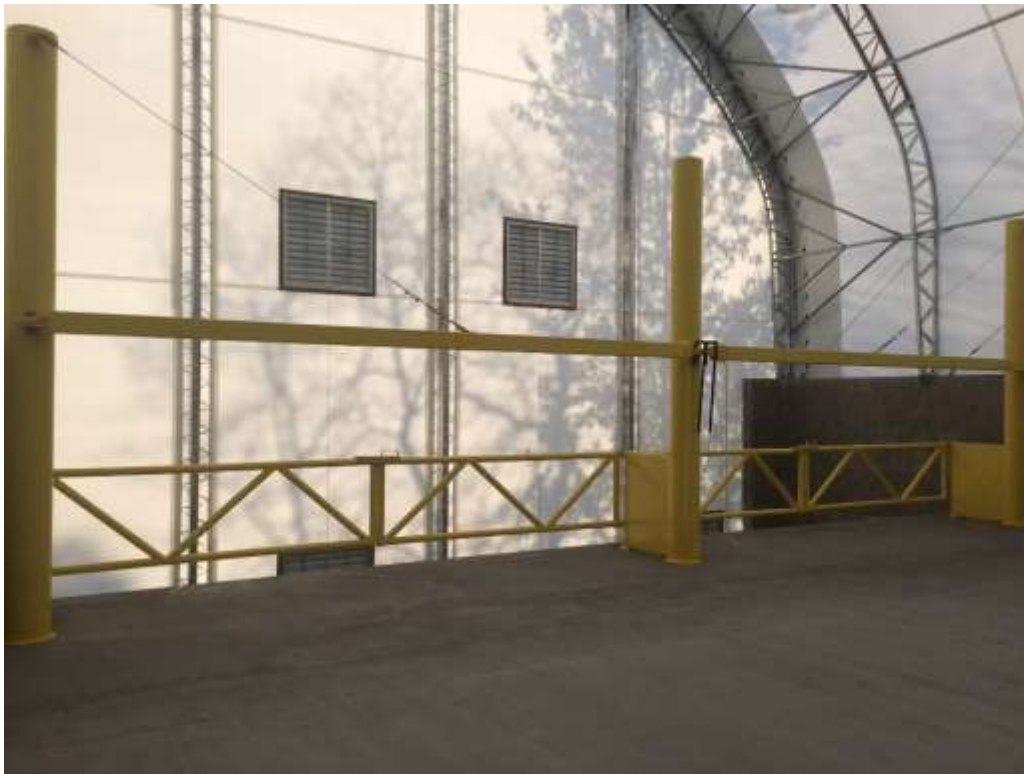
Photo 1: Example of Transfer Station Safety Rails
