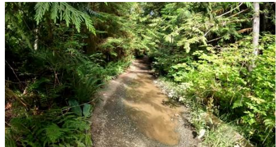
Figure 12. Drainage and trail upgrades needed.
