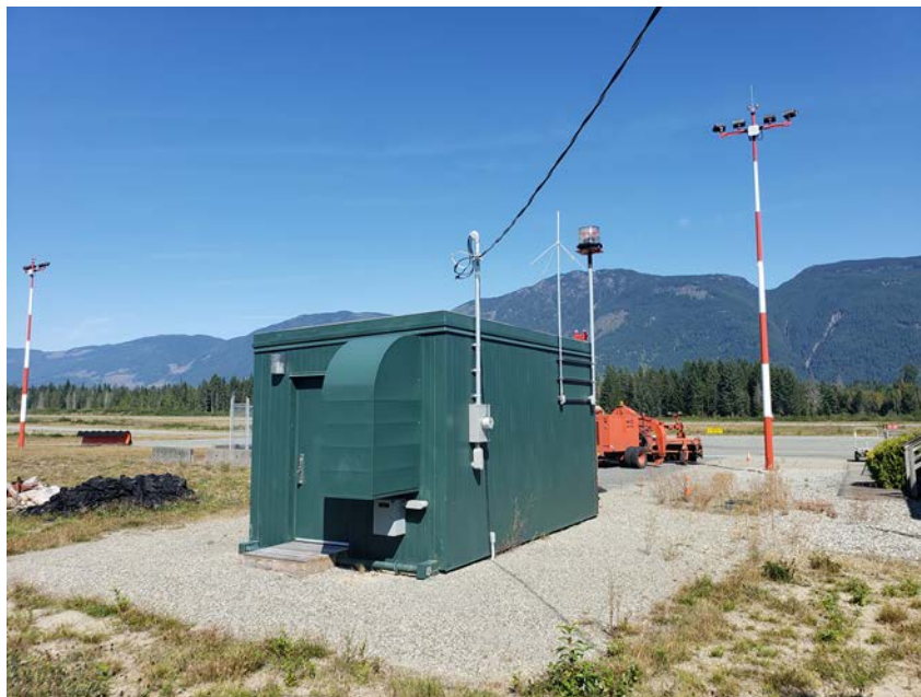
AVRA Lighting System
