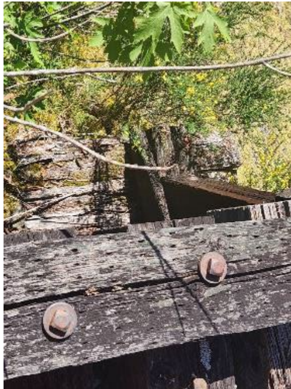
Figure 3-48: Bridge at Mile 25.0 – Mud Sill Decay
