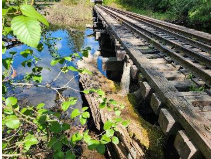
Figure 3-44: Bridge at Mile 22.1 – Debris Build up in North Side
