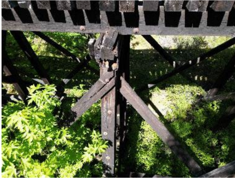
Figure 3-49: Bridge at Mile 25.0 – Failed Cap and Brace
