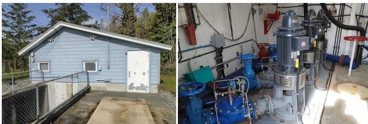
Figure 27. Exterior and interior of the McKenzie Rd pump station.
